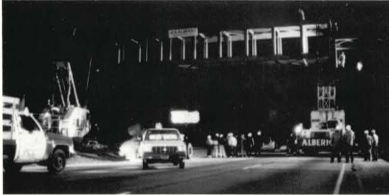
An early-hours "SPAN-DEMONIUM" party marked placement of the last span in the Smith Bridge across Highway 44.
